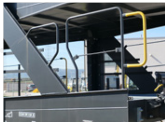
All handrails separately attached, some made of metal
